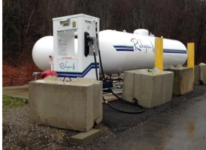
Figure 10 – Propane Fueling Station at Customer Site
