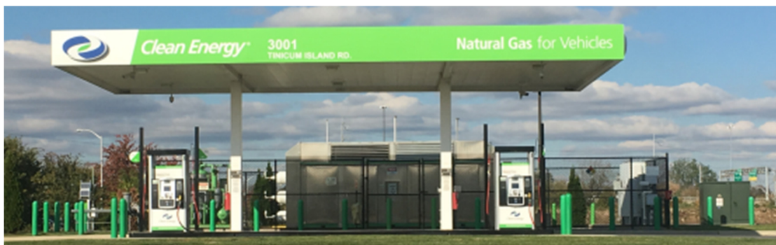
Figure 8 – “Wally Park” CNG Fueling Station at Philadelphia Airport
