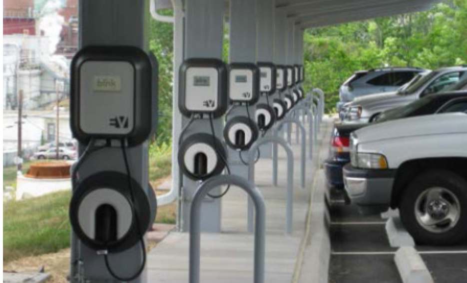
Figure 11 – Level II Fleet Charging Stations
