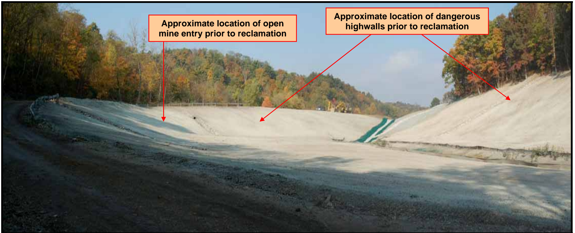
Figure 9 – Panoramic views of reclaimed Fishing Run project site showing re-contoured highwalls and re-constructed Fishing Run stream channel.
