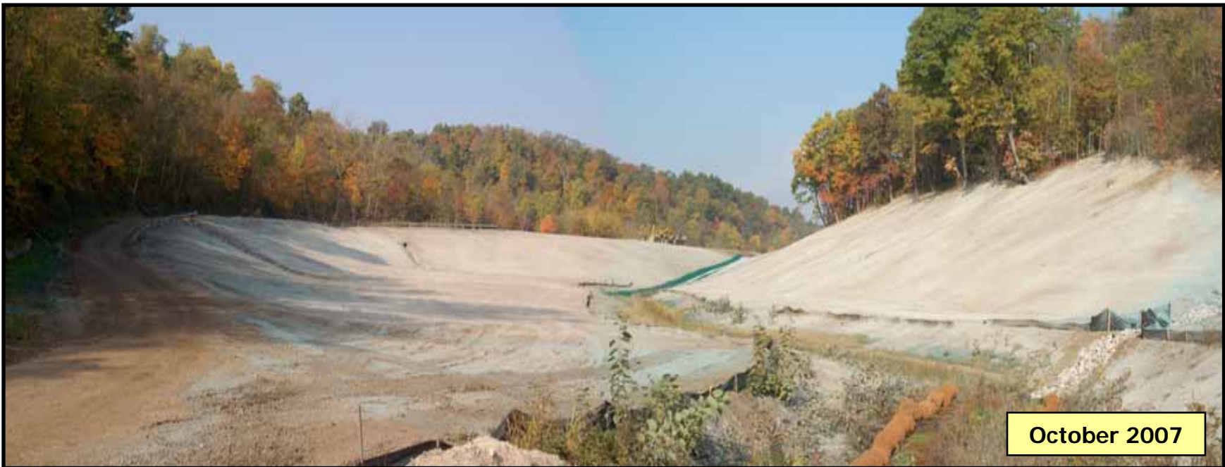
Figure 6 – Site from lower end at initiation of construction (above) and near completion of construction (below).
