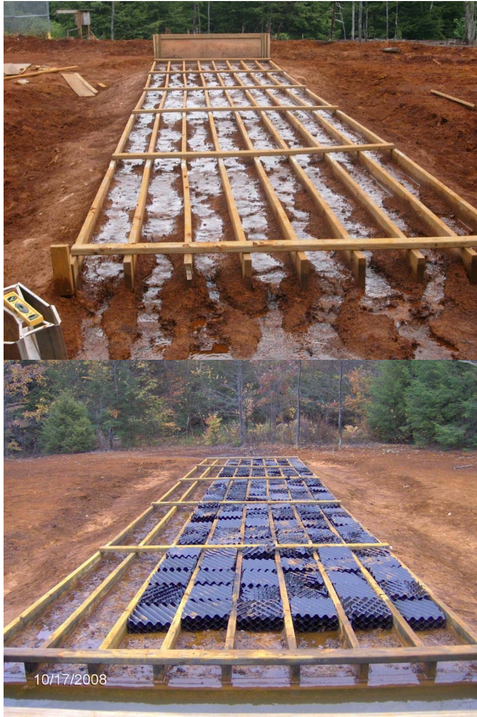
Figure 3. Photos of pilot-scale experimental facility constructed on the Hughes Borehole iron mound. Water is conveyed from primary discharge channel through a 3-inch PVC pipe into the “splitter” box and then into eight, 40-foot long channels. Upper photo (looking uphill) was taken in June 2008 shortly after construction. Lower photo was taken in October 2008 after installation of plastic filter media in six of the eight channels (looking downhill). Channels are identified from right to left in the upper photo (i.e. upstream view) as A – H.
