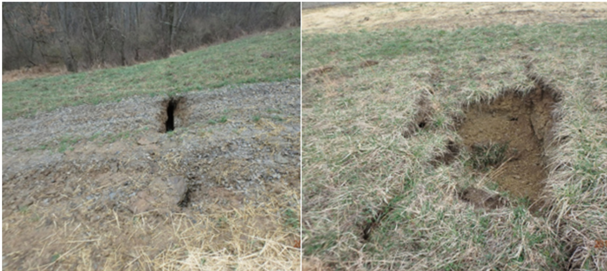
Figure 6-2. Tension cracks formed during undermining of a property in the Bailey 3L panel (Photographs from the PADEP files).
