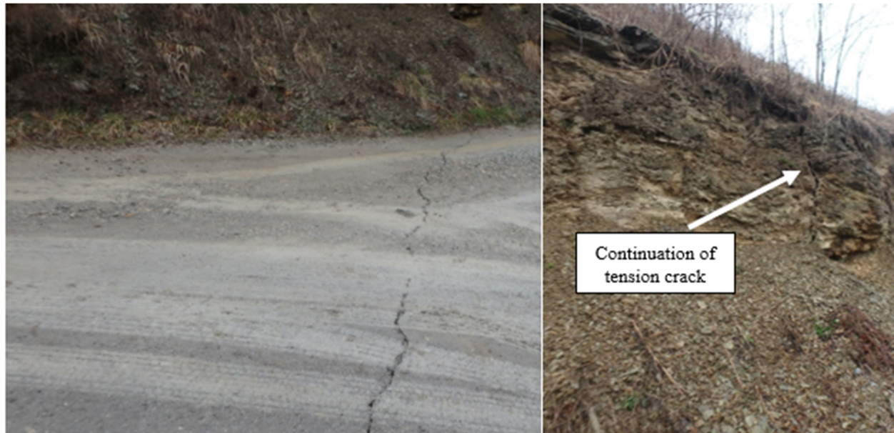
Figure 6-3. Tension cracks in roadway and hillside formed a month after the Bailey 5L longwall face had passed (Photographs from the PADEP files).
