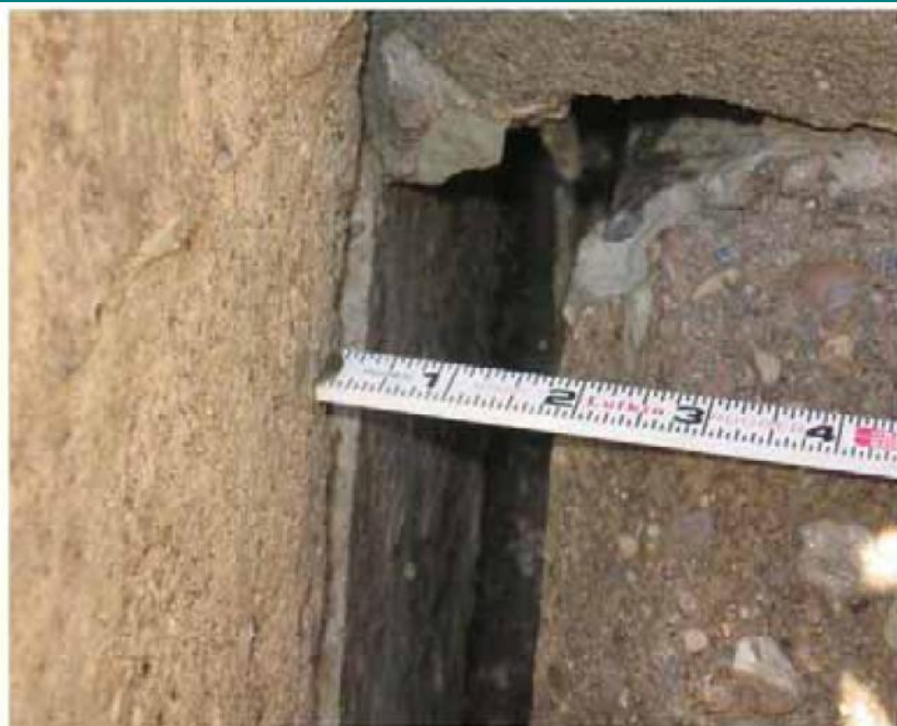
Photo 2. Open Joint between Right Non-Overflow and Spillway (Photo December 2006)
