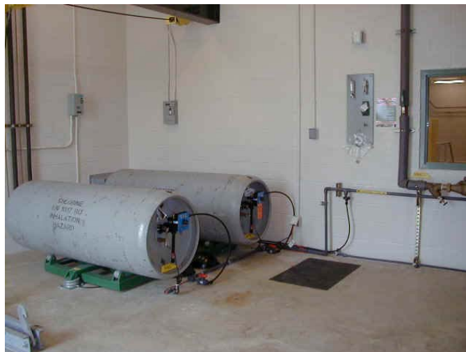
Figure 2.2 Ton Cylinders in Feed Position
