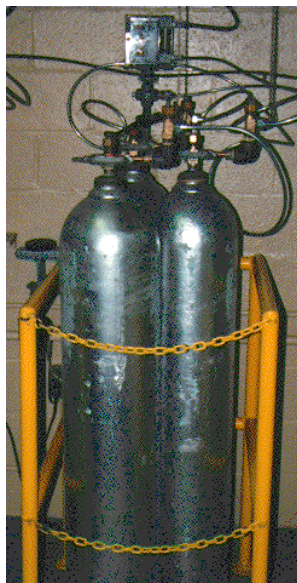
Figure 2.1 A 150 lb Chlorine Cylinder in Feed Position
