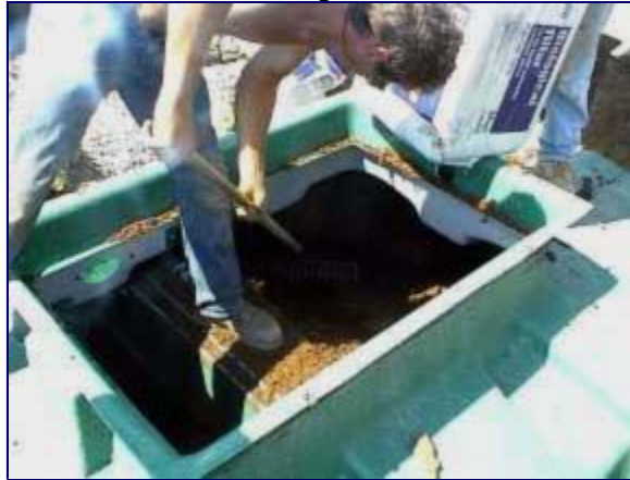
Ecoflo Unit Being Filled with Peat
