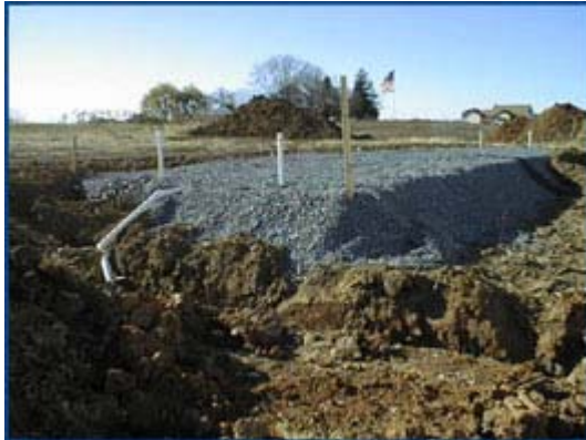
At-Grade Absorption Area
