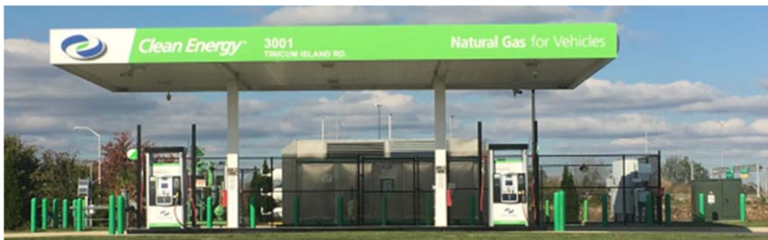
Figure 7 – CNG Fueling Station at Philadelphia Airport
