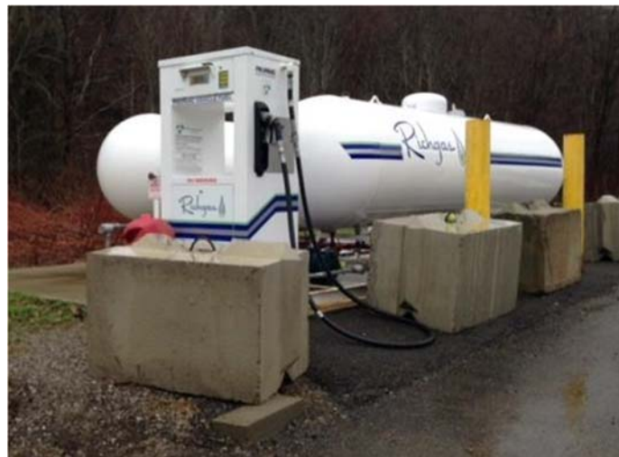
Figure 9 – Propane Fueling Station at Customer Site
