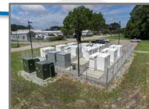
Battery System 4 MW / 8 MWh Capacity
