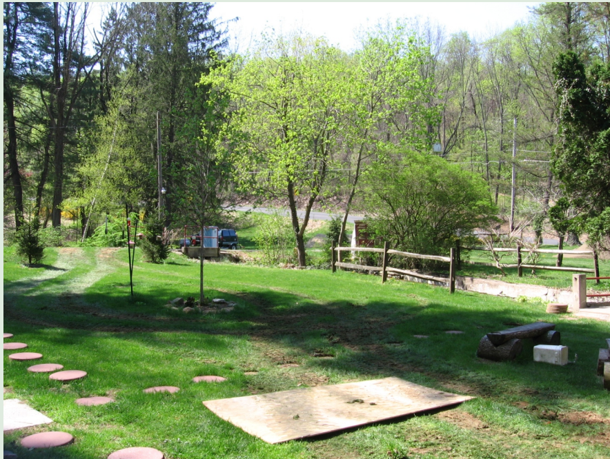
Restoration is almost complete in 2015 at the Mt. Laurel Road Battery Casing Site, Alsace Township, Berks County, Pennsylvania.
