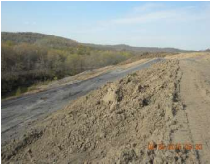
Grading of soil covering material on terraced face above creek facing southwest.
