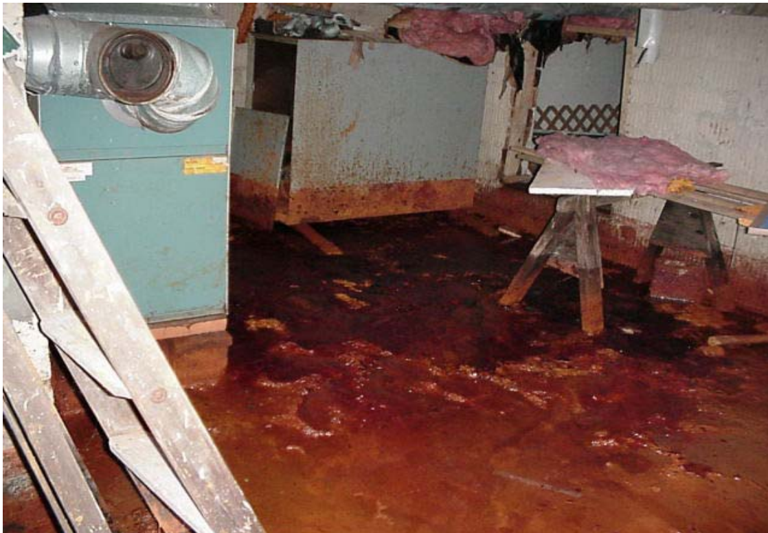
Figure 1: AMD in home basement Village of Melcroft
