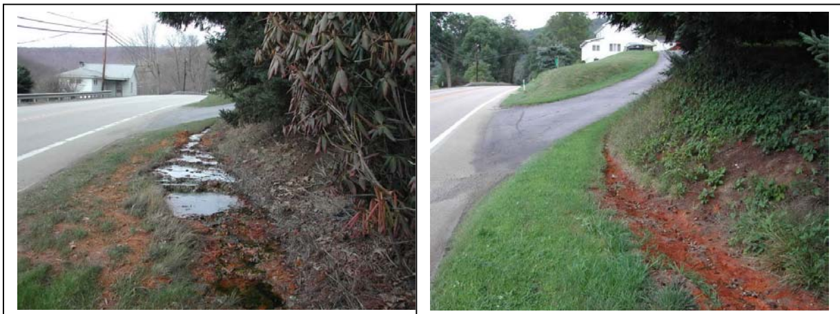
Figure 5: Typical cropline discharge area before and after dewatering
