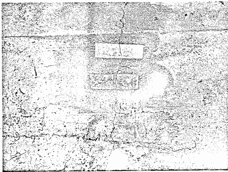
Fig. 2—Paper "telltale" used for indicating movement of old cracks. Second "telltale" was applied after first was partially torn.
