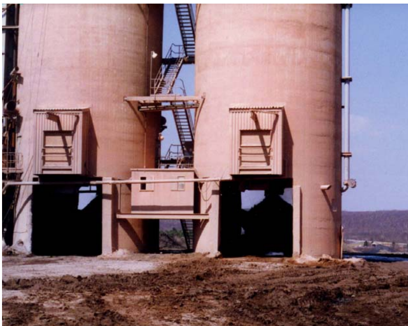
Figure 9.7. Fly and bottom ash silos for storage until placement on the NEPCO site.
