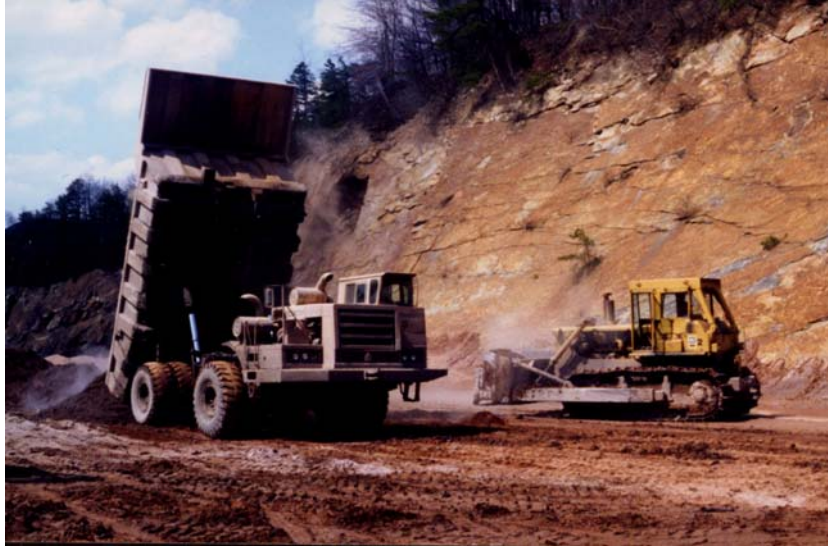
Figure 9.8. A truck and bulldozer used to transport and place ash in the Big Gorilla mine pool.
