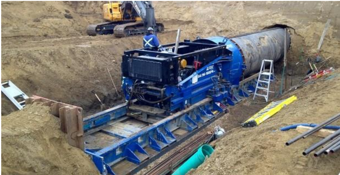
Figure 2: Typical CAB Entry Pit Workspace Area – Photo
