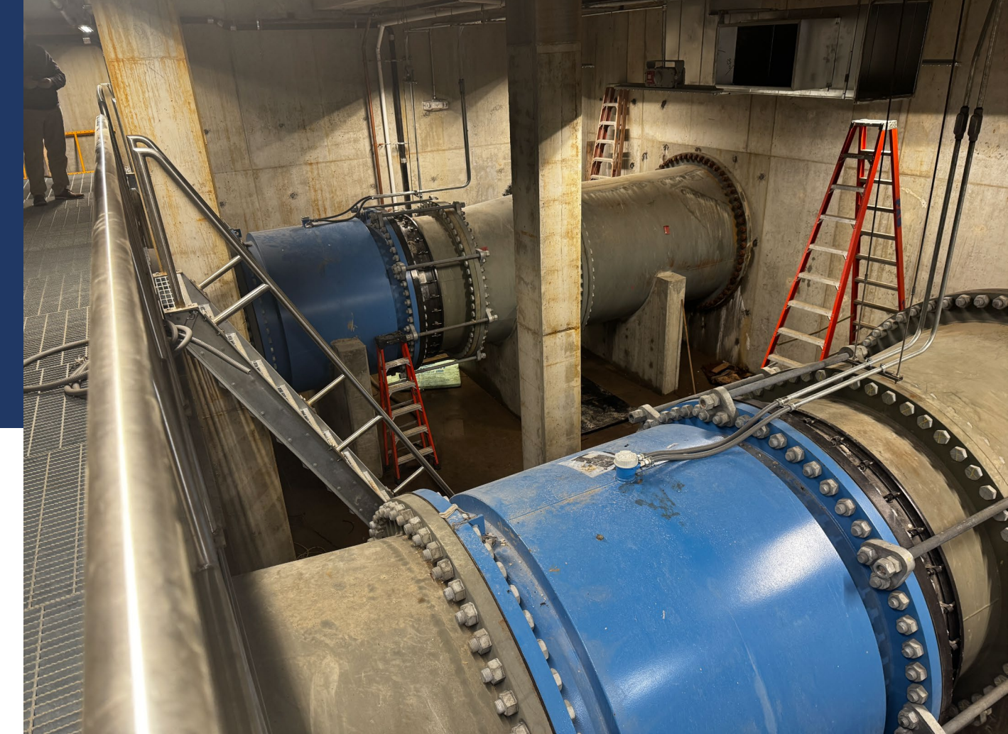
NE Prelim Treatment Building Conduits
