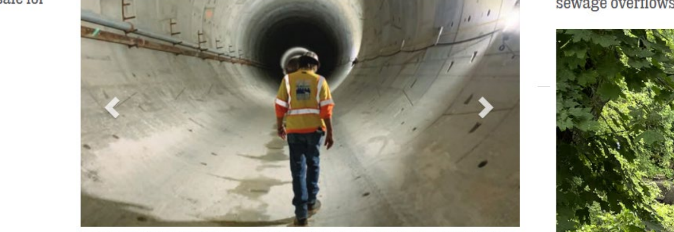
Washington, D.C.'s Northwest Boundary Tunnel before its opening in September 2023. The five-mile-long, 23-foot diameter tunnel reduces about 98% of sewage overflows into the Anacostia River each year, according to DC Water, and can also reduce flooding by 7 to 50% in a given year.
