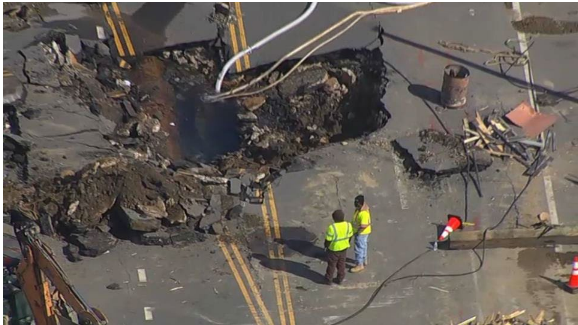
Conditions after 48" transmission main break – Philadelphia, PA (Photo from NBC10)
