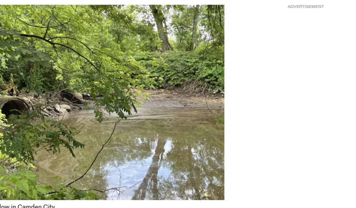
A combined sewer overflow in Camden City. Frank Kummer
