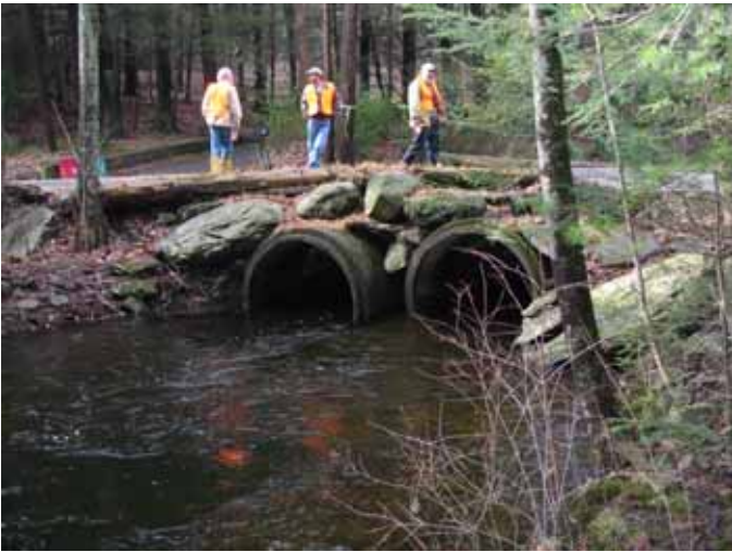
Figure 8 - Cranberry Creek at Cranberry Creek Road crossing. Culvert undersized, road frequently floods. Stream receives a large amount of road runoff. Non-point source pollution management recommended here.
