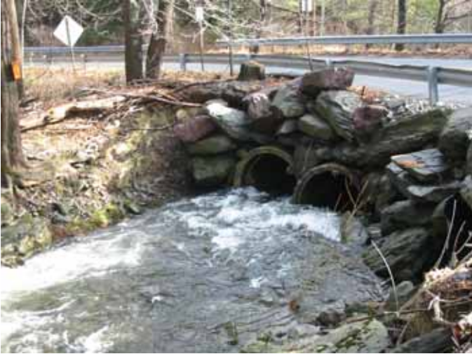
Figure 7 - Cranberry Creek at Browns Hill Road: culvert is undersized, threatens road. Culvert should be replaced and sized sufficiently to provide additional cross sectional area and improve fish passage.
