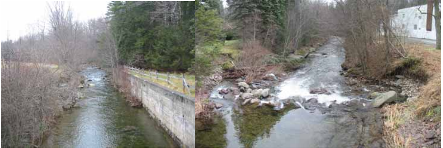
Figure 20 – Upper Paradise Project 2: Pocono Gardens Resort Site – upstream view of channelized section (above) and downstream view past breached dam (right).
