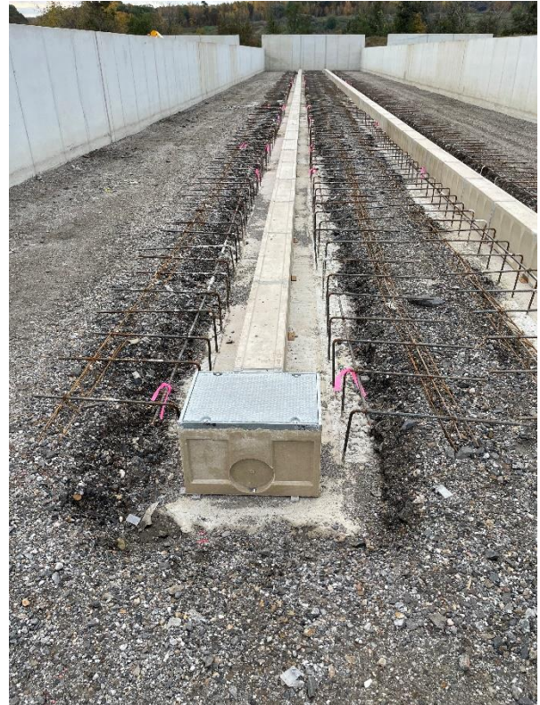
Aeration-Moisture Removal Channel Installed
