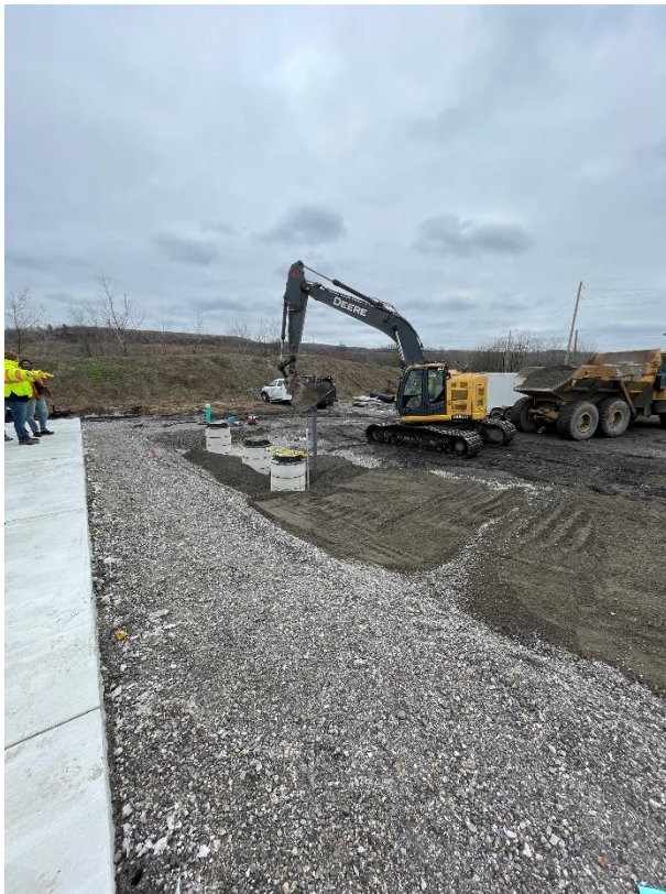
NSP Gore Bunker Leachate Storage Tanks 5Dec2023
