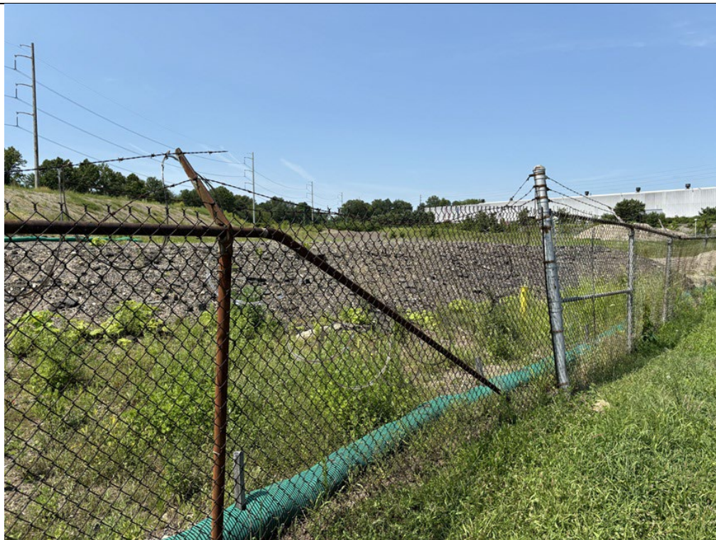
Section of damaged security fence along 51 st St.
