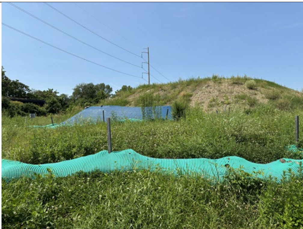
Contaminated fill dirt stockpile covered by blue tarp, with filter sock in foreground.
