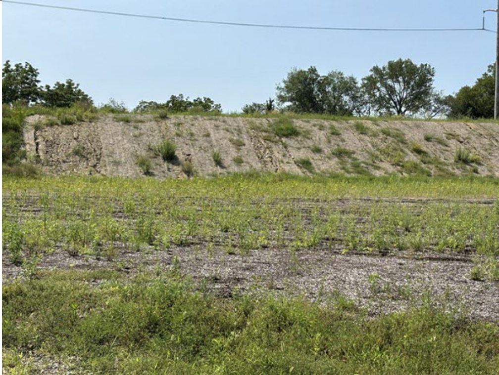
Downslope portion of large fill dirt stockpile, with significant erosion present.
