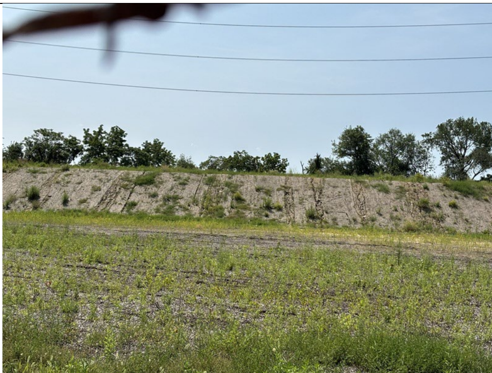
Large fill dirt stockpile, with erosion rills and gullies present.
