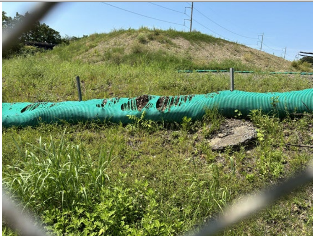
Filter sock at downslope border of site showing wear.
