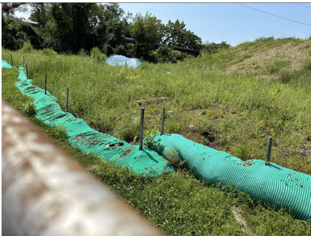
Filter sock at downslope border of site showing wear.
