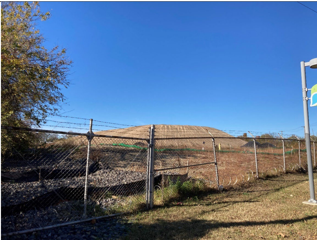
Downslope end of large fill dirt stockpile, taken from Bartram's Garden trail.
