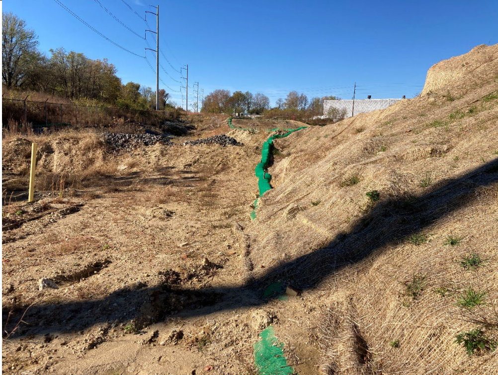
Filtersock (with overtopping) looking upslope along southern end of large fill dirt stockpile. One stone check dam is visible in swale towards upper left.
