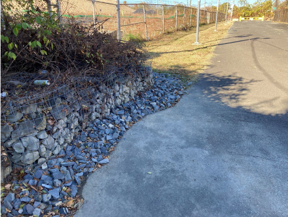
Sediment staining along Bartram's Garden trail.
