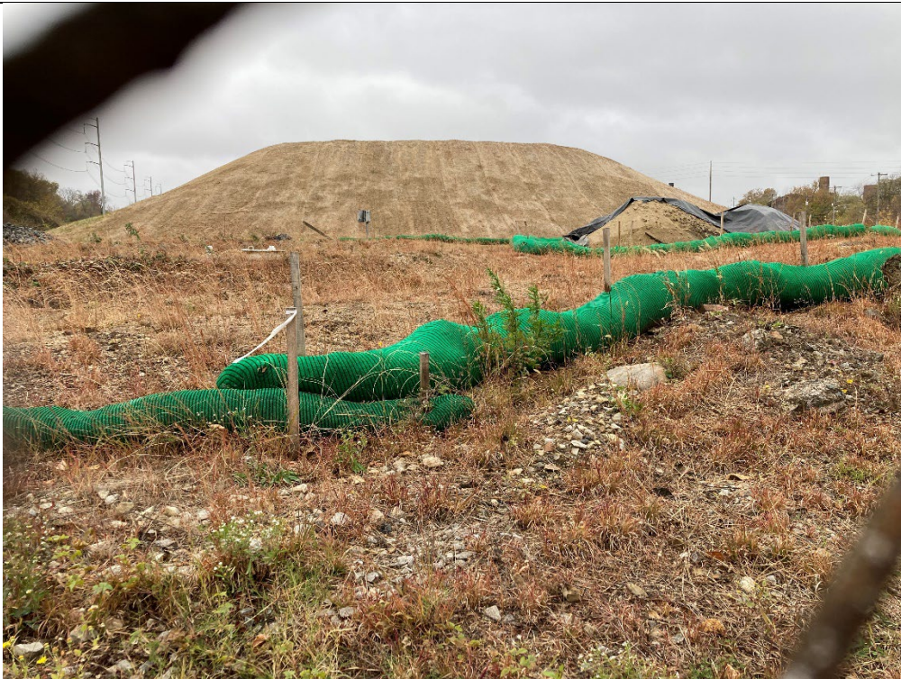
Large fill dirt stockpile with gullying present in background, with partially exposed contaminated dirt pile in front.
