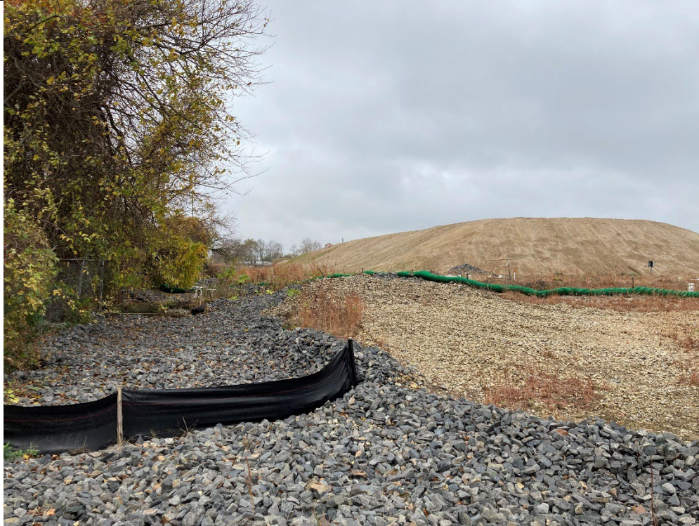
South side of large fill dirt stockpile, with silt fence in foreground, taken from Bartram's Garden trail.
