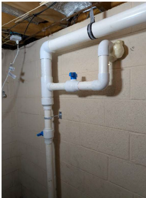
Vertical and horizontal extraction point
