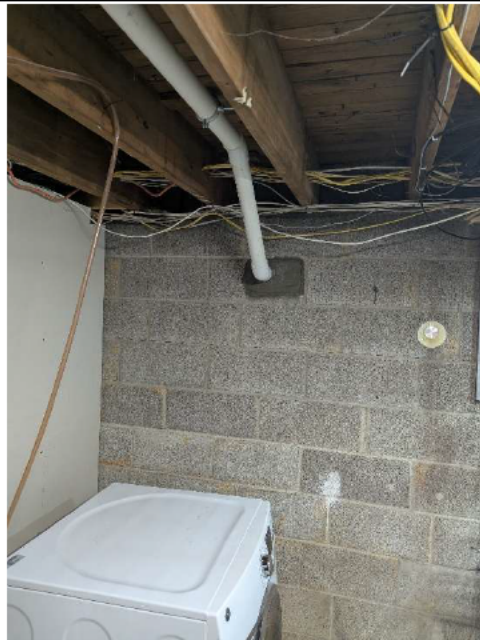
Horizontal extraction point and vapor pin
