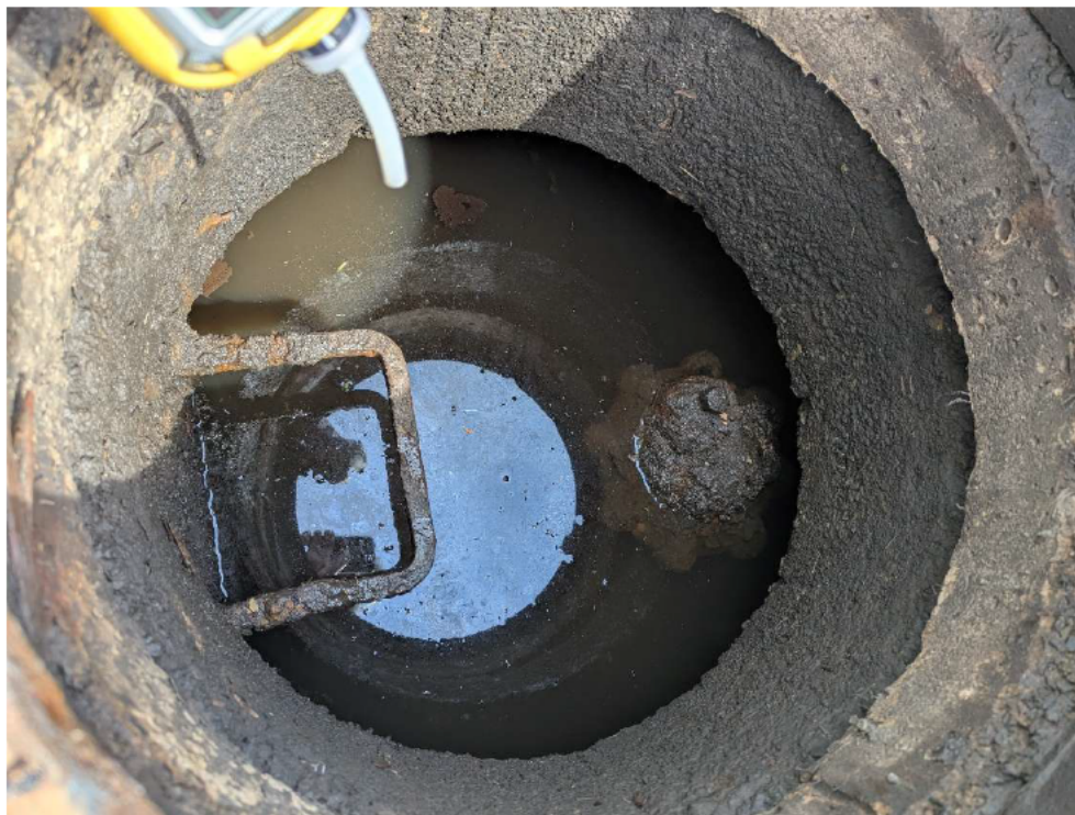
Water with sheen in ARV vault
