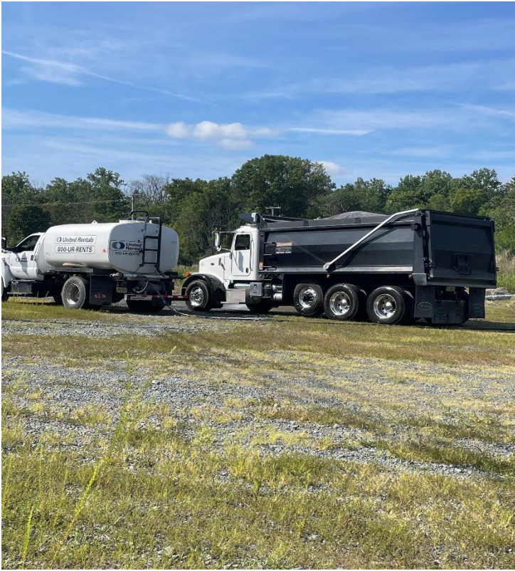
Water truck being used to wash the wheels of the truck-8/22/23, 1024am
