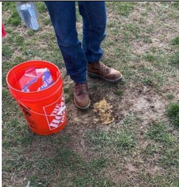
Hole is backfilled with clean sand, then remaining native soil placed on top. 3/17/2025 @ 1630
