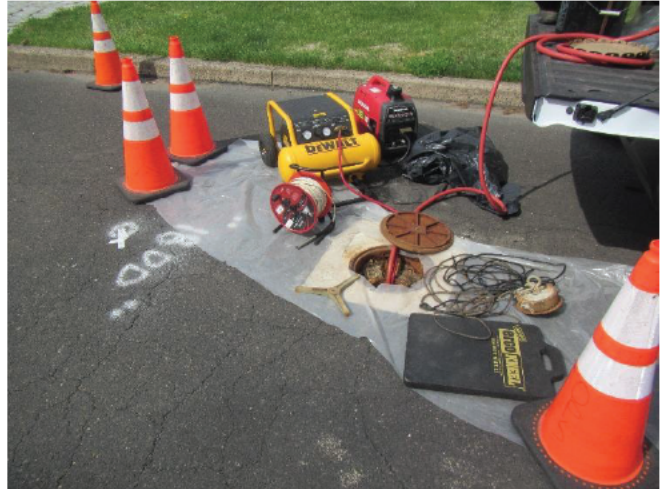
Pumping setup at RW-2 with proposed MW-18DD visible.
