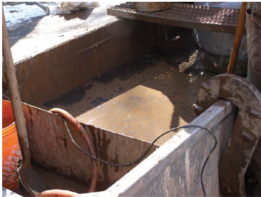
Recovered groundwater with black organic material 2-25-26 @ 12:08
