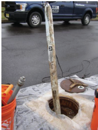
Pulled absorbent sock from recovery well RW-3 in Glenwood Drive 3-23-26 @ 9:45
