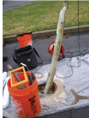
Pulled absorbent sock from recovery well RW-2 in Glenwood Drive 3-23-26 @ 9:33
