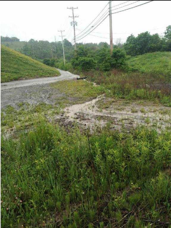
Flow not making it to drainage swale at Outfall 021
