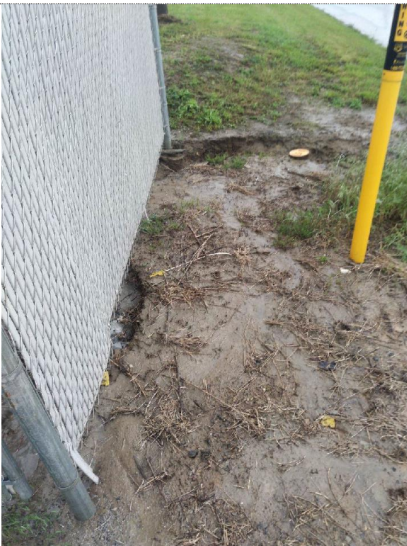
Erosion downstream Columbia gas site vicinity Outfall 021
