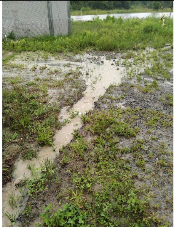
Erosion upstream of Columbia gas site vicinity Outfall 021
