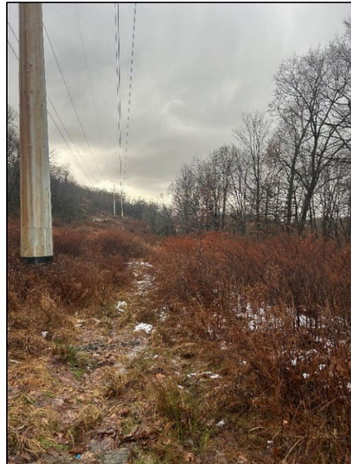
Transmission lines running through the site
