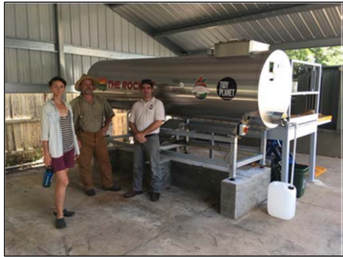
In-Vessel composting system
