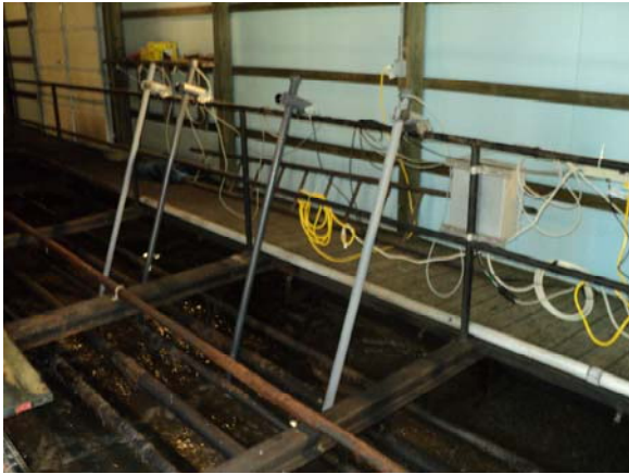
Figure F.1: MLSS and pH probes, East Oxidation Ditch
