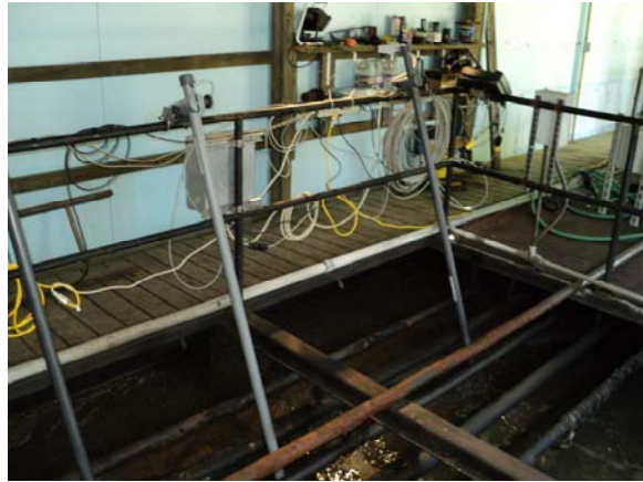
Figure F.2: DO, ORP, and Nitrate probe placement
