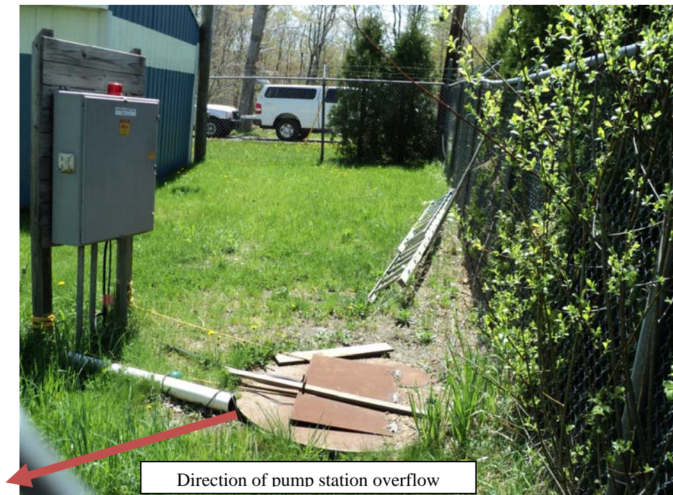
Figure F.8 Influent Pump station
