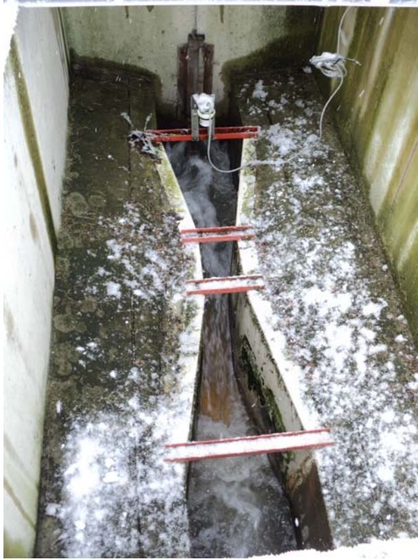
Figure F.7: Effluent flow meter and discharge flume
