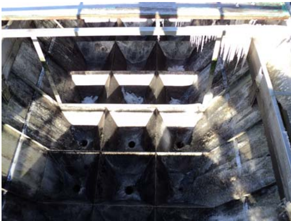
Figure F.9: Bottom of boat clarifier after draining; note return sludge ports
