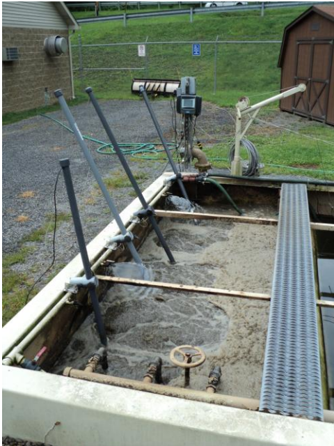
Figure C.1 Locations of ORP, DO, MLSS, and pH probes in the aeration tank
