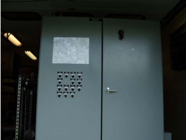
Figure G-7: PLC Control Panel
