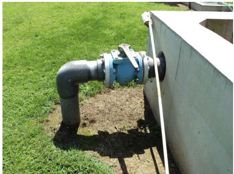
Figure G-12: Recycle Sludge Valve
