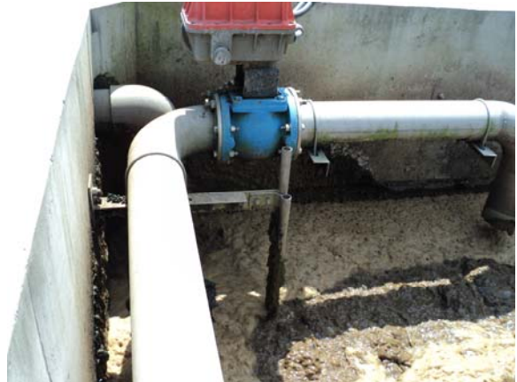
Figure G-19: Problematic Automatic Valve
