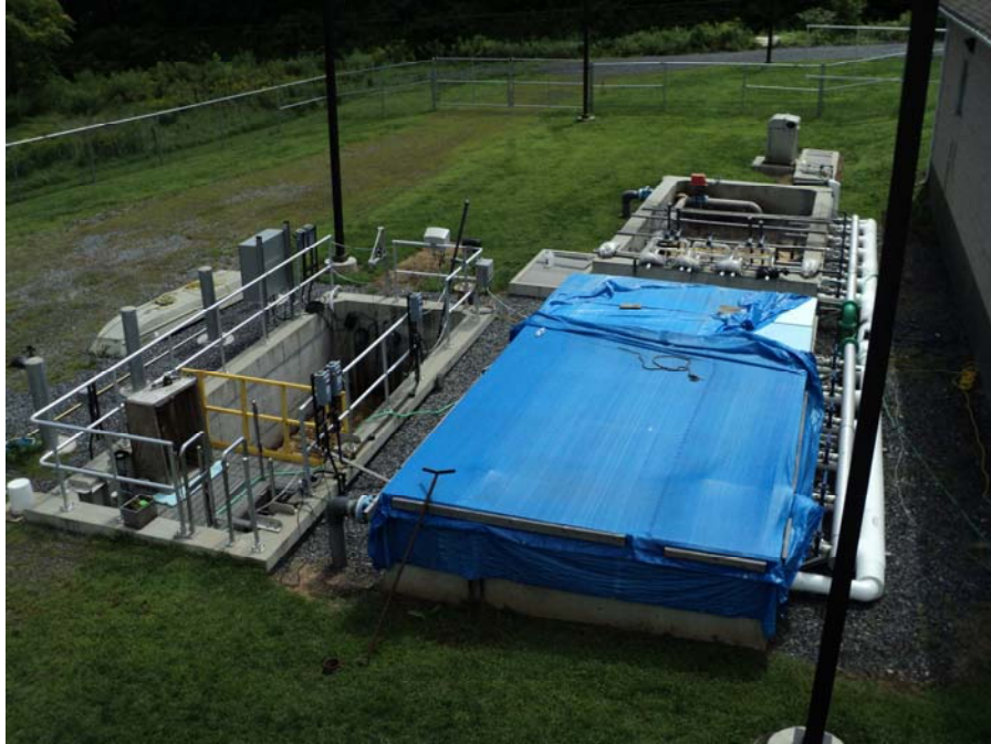
Figure G-1: Portland Treatment System: Anoxic Tank (left); MBRs (right); Freshening (upper right)
