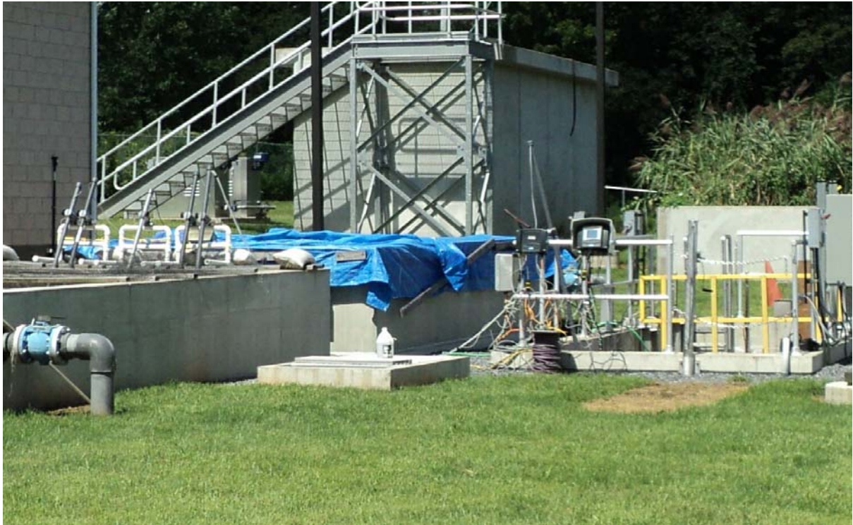
Figure G-13: Hach SCADA Equipment Mounted in Process Tanks
