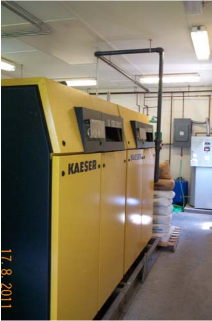
Figure G-3: MBR Blowers
