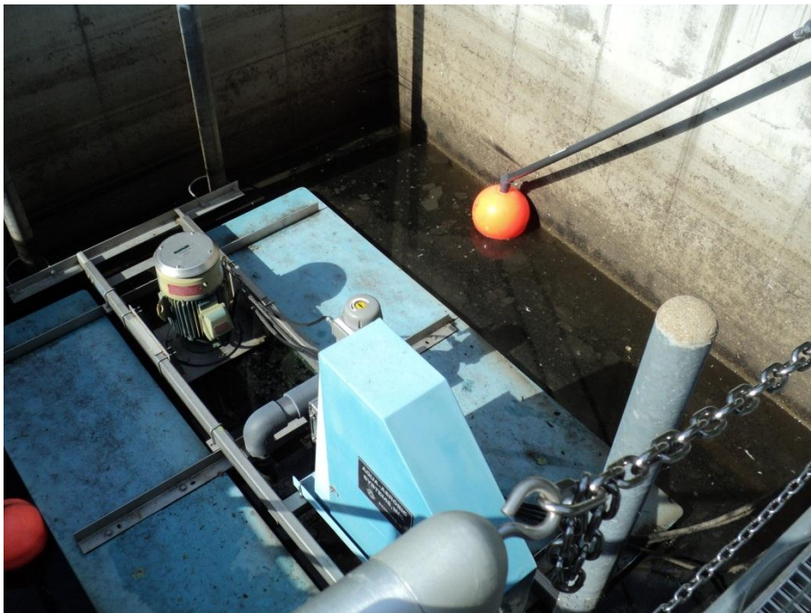
Figure B.3: Photo showing example of online monitoring equipment installed in the SBR at the PI plant.
