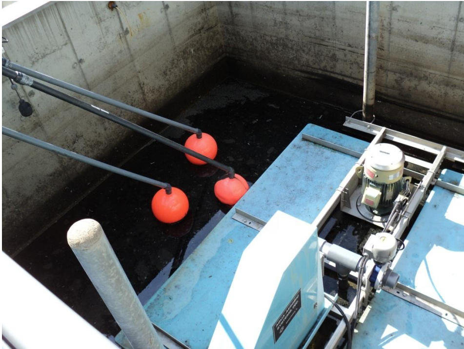
Figure B.2: Photo showing example of online monitoring equipment installed in the SBR at the PI plant.
