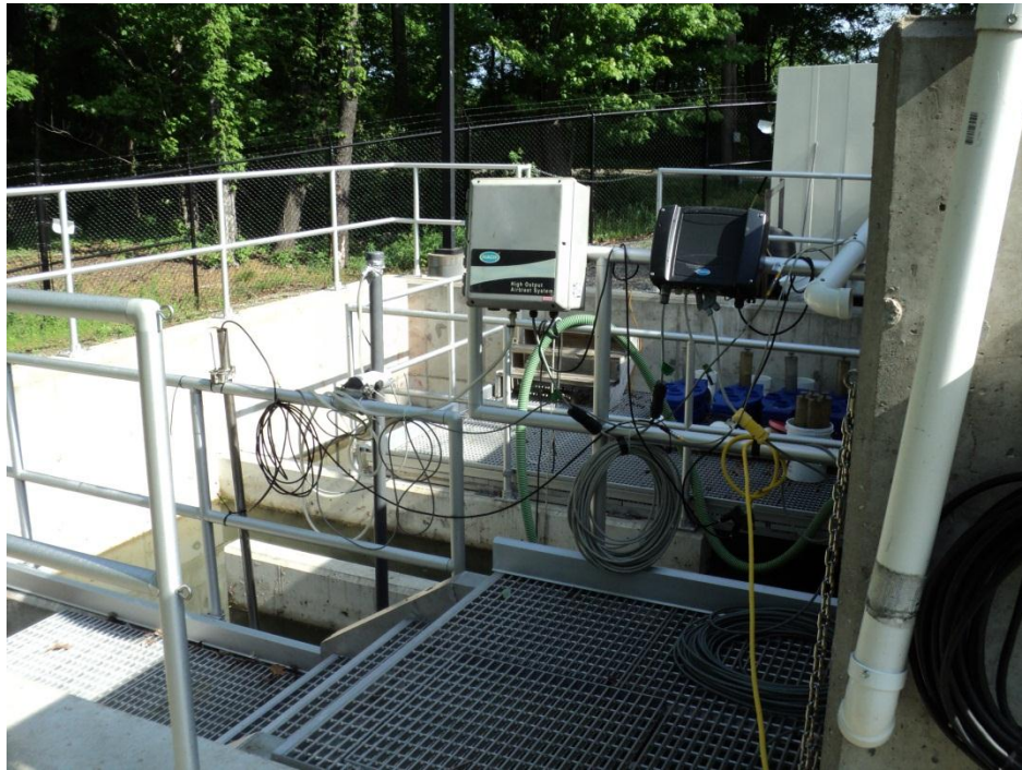
Figure 5: Chlorine contact tank area with nitrate and ammonia probes installed.
