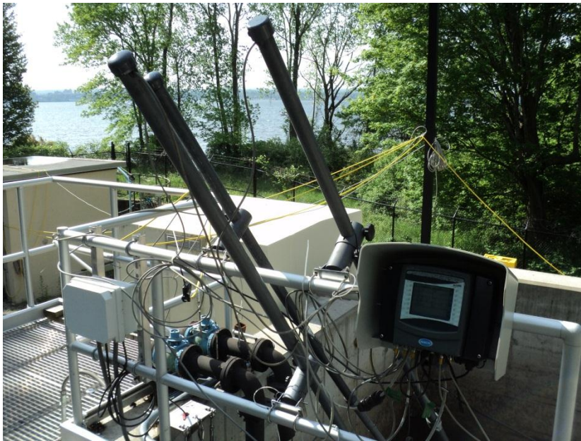
Figure B.1: Photo showing example of online monitoring equipment installed at the PI plant.
