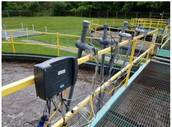
SC controller & Sensor Probes at Unit 1
