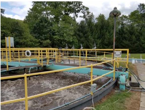
Rigging / Power for Anoxic Grinder Pump, Unit 1
