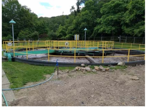
Unit 2 Reactor in C/S Mode
