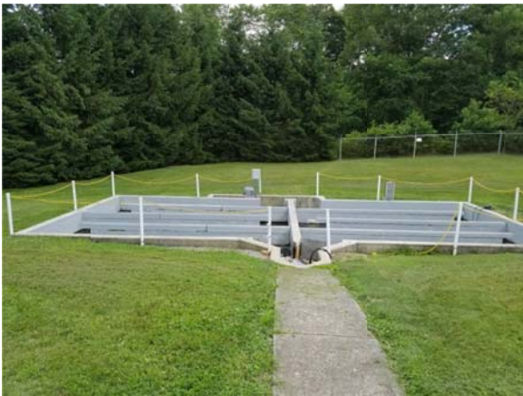
Disinfection Contact Tanks
