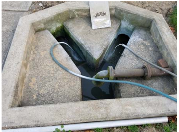
Secondary Splitter Box, w/ Mg(OH) 2 feed to both units
