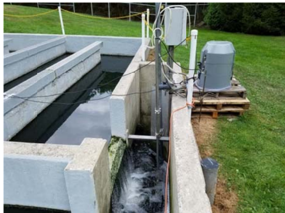
Final Effluent NH4 & NO3 Probes & Composite Sampler
