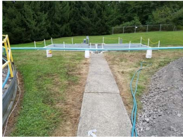
Temporary WAS line, Unit 1 to Unit 2 Sludge Holding
