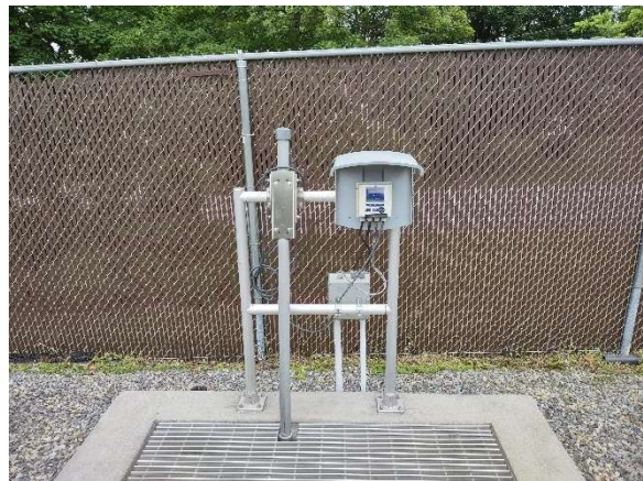
D.O. Probe & Controller for aeration VFD
