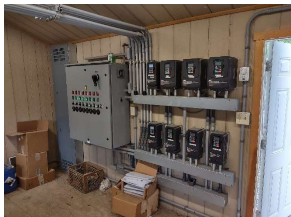
Control Panel & VFDs
