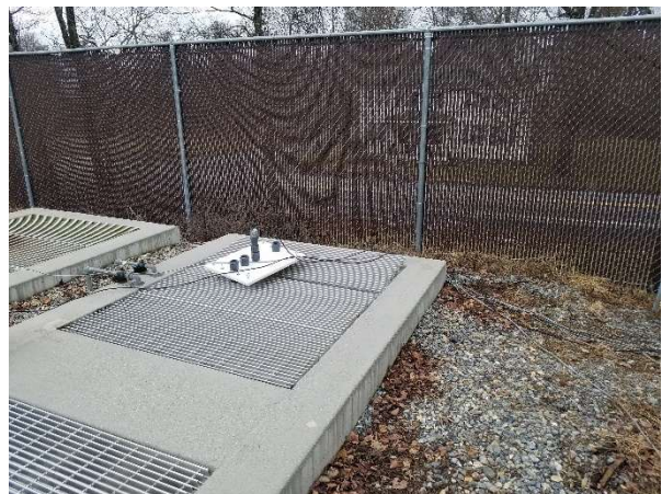
UVAS probe at splitter box
