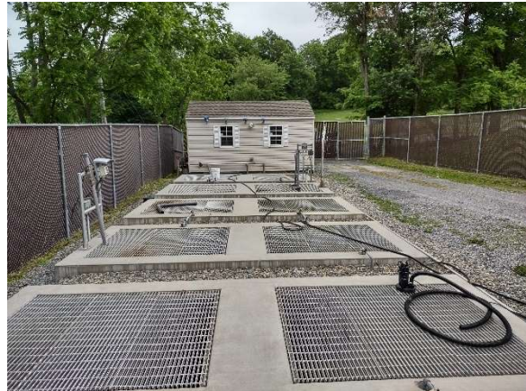
Wastewater Treatment Facility
