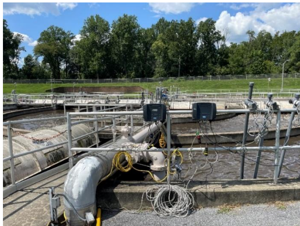
Figure B-3: Photo of HACH pH, D.O., ORP, and MLSS continuous monitoring probe and SC1000 controller installation location in the AMITY WWTF oxidation ditch treatment units.
