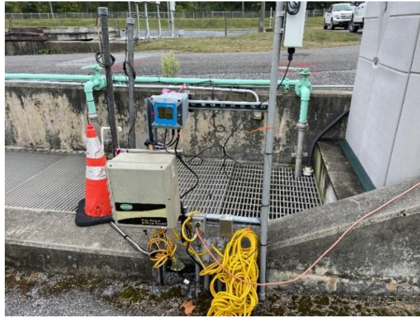
Figure B-7: Photo of HACH SC4500+ controller, airblast unit compressor (for AISE probe), and Nitratax & AISE probe installation location in the WWTP effluent trough. The new SC4500+ controller was installed on September 17 th , replacing the SC1000 controller and universal display.
