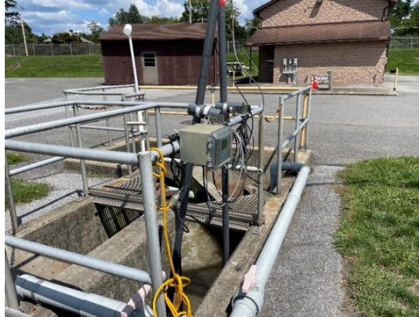
Figure B-1: Photo of HACH UVAS and pH continuous monitoring probe installation location in the AMITY WWTF influent trough from August 21 st through October 23 rd , 2024.
