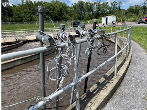
Figure B-4: Photo of HACH pH, DO, ORP, and MLSS continuous monitoring probe installation location in the AMITY WWTF oxidation ditch #1 (outer) treatment unit.
