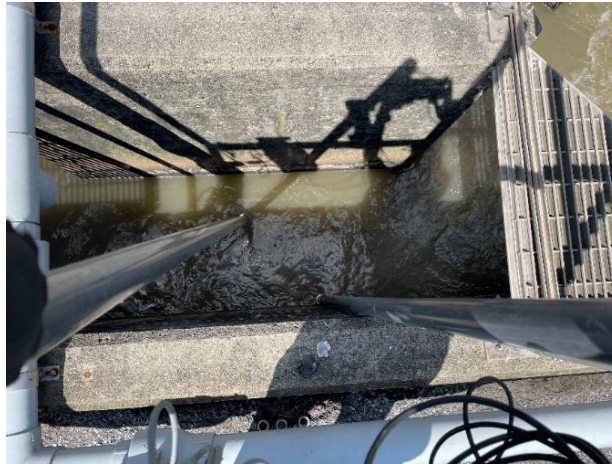
Figure B-2: Photo of UVAS continuous monitoring probe installation location in the AMITY WWTF influent trough after the influent screening and grit removal processes.
