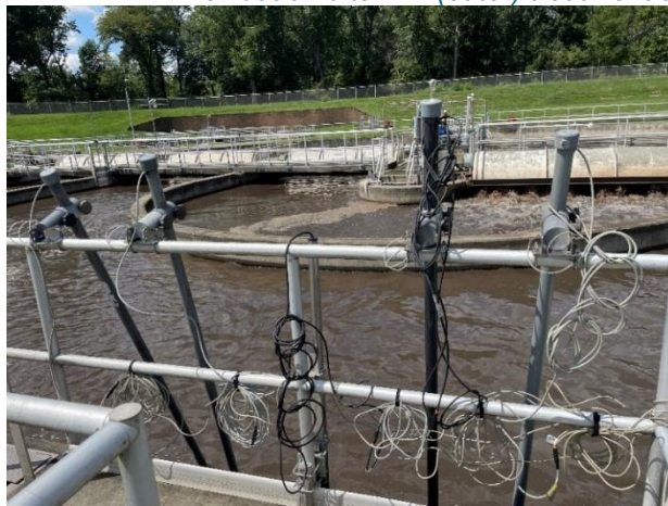
Figure B-5: Photo of pH, DO, ORP, MLSS, and nitrate-nitrogen continuous monitoring probe installation location in the AMITY WWTF oxidation ditch #2 (middle) treatment unit.
