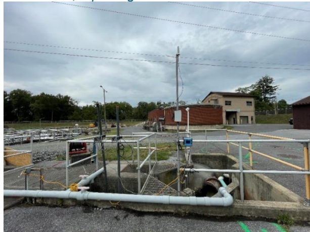
Figure B-8: Photo of HACH SC4500+ controller and pHD & UVAS continuous monitoring probe installation location in the Amity WWTP influent trough.
