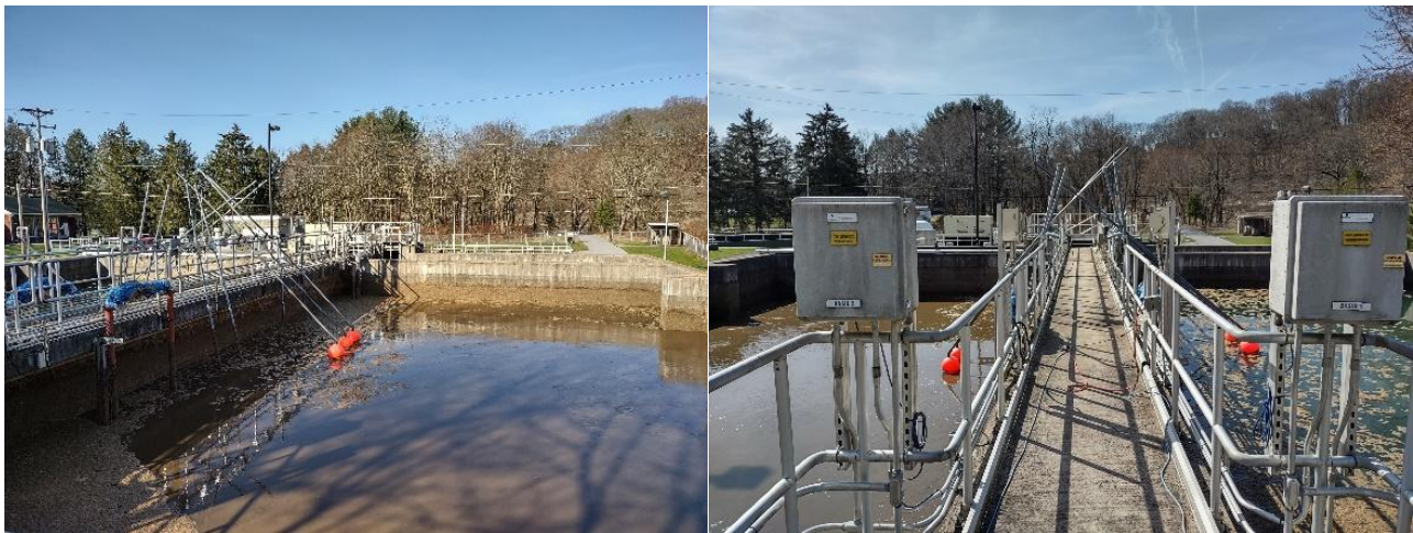
Figure B-2 & B-3: Photos of WWTAP continuous monitoring equipment installation locations in the Curwensville WWTF SBR treatment unit tanks.
