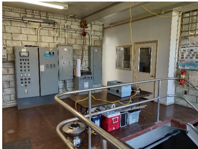
Figure B-8: Photo of PADEP WWTAP process control & bench testing laboratory at Curwensville WWTF.
