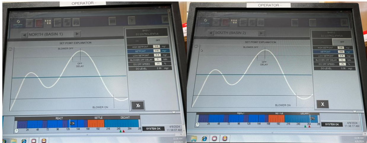
Figure 2. Photographs of the WWTF Sanitaire/Xylem SCADA system user interface for SBR treatment unit aeration blower control setpoints.
