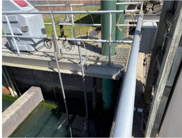
Figure B-6: Photo of HACH Nitratex ( n\text{NO}_3\text{-N} , nitrate) and HACH AISEsc ( \text{NH}_4\text{-N} , ammonium) probe installation location in the Curwensville WWTF final effluent chlorine contact tank from March-May 2024.
