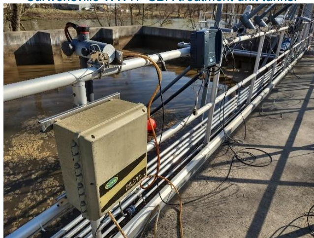
Figure B-4: Photo of continuous monitoring probe mounting installation location in the Curwensville WWTF SBR treatment unit tanks.
