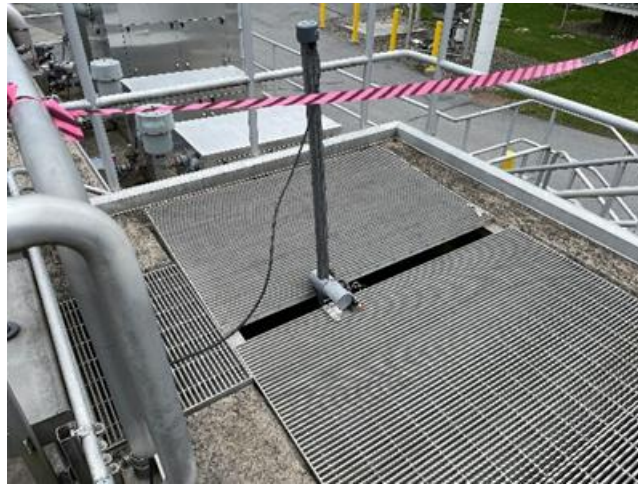
Figure B-1: Photo of UVAS continuous monitoring probe installation location in the Curwensville WWTF.
