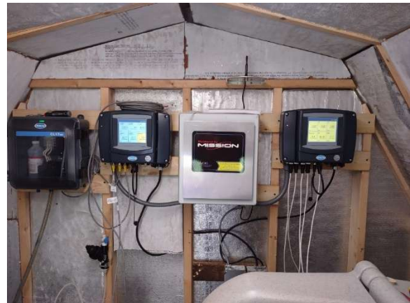
Photo 3: Hach probe controllers, the CL17 TRC miniaturized lab, and the Mission Systems telemetry connection.
