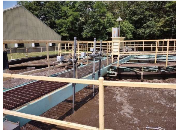
View of probes “permanently” installed by Jenner’s telemetry contractor
