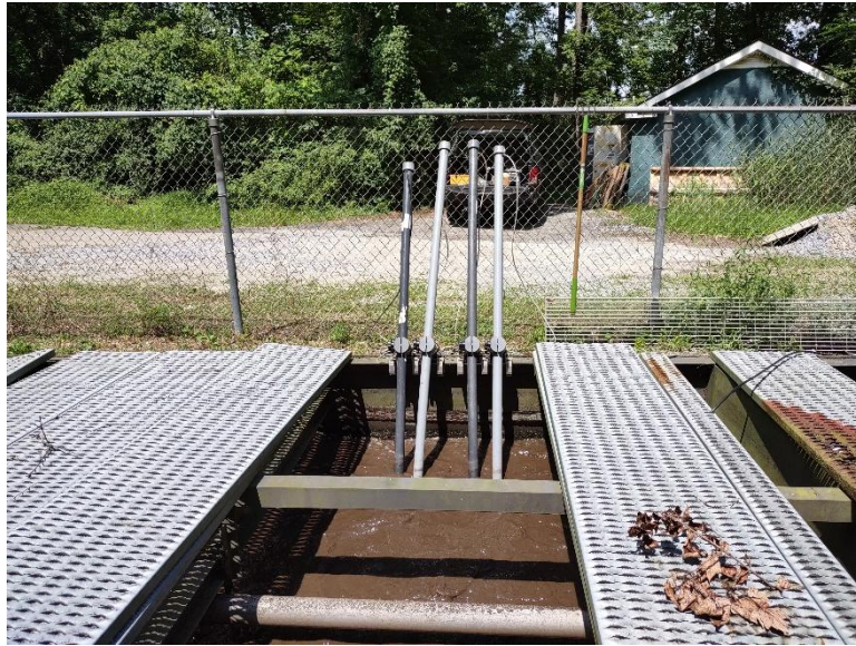
Figure 11: WWTAP pH, DO, ORP, and Solids continuous-monitoring probe installation in RRMSA WWTF Aeration Tank #1.
