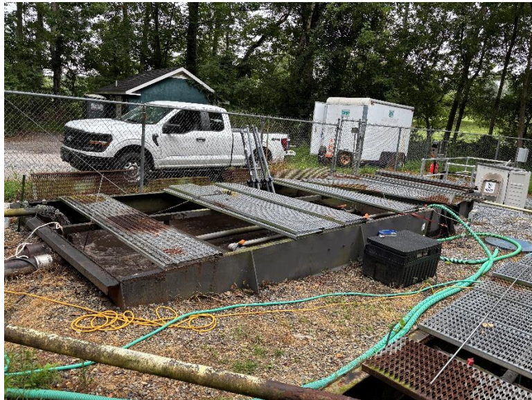
Figure 12: WWTAP pH, DO, ORP, and Solids continuous monitoring probe installation in RRMSA WWTF Aeration Tank #1.
