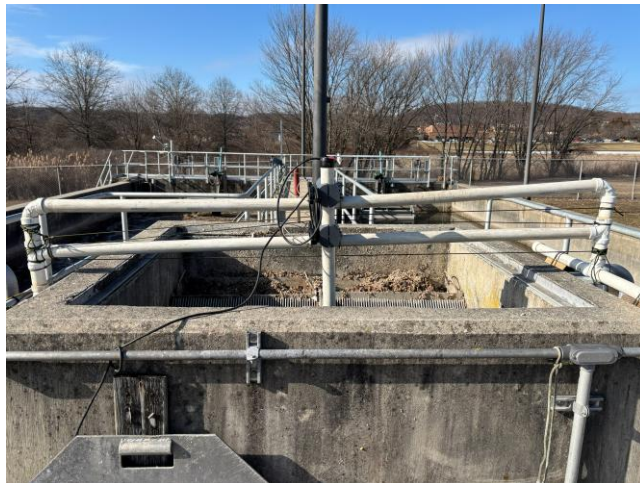
Figure B-2: Photo of UVAS continuous monitoring probe installation location in the WWTF influent distribution box.
