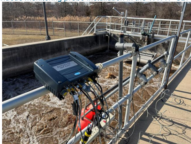
Figure B-6: Photo of continuous monitoring probe installation location in the WWTF SBR#2 treatment unit (react).
