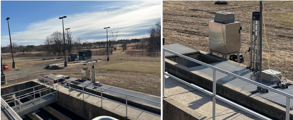
Figure B-7: Photo of HACH SC4500+ controller, airblast unit compressor (for AISE probe), and Nitratex & AISE probe installation location in the WWTP effluent trough.
