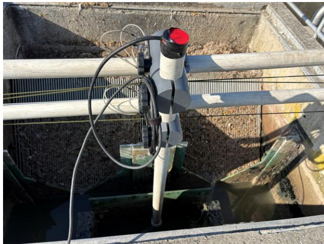
Figure B-3: Photo of UVAS continuous monitoring probe installation location in the WWTF influent distribution box.
