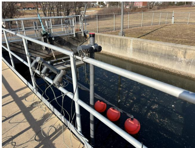
Figure B-5: Photo of continuous monitoring probe installation in the WWTF SBR#1 treatment unit (settle).
