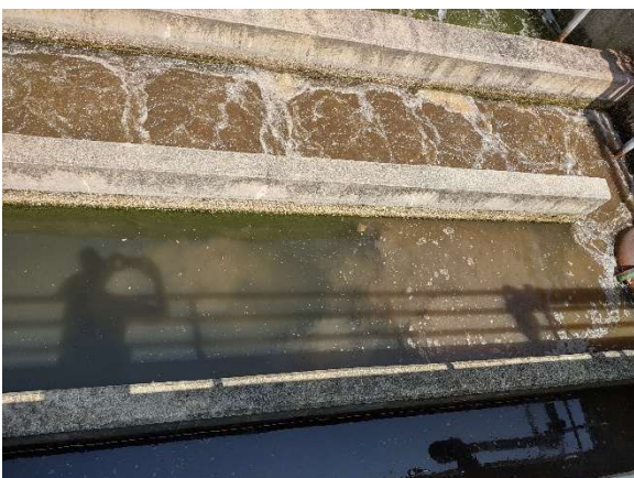
Suspended solids in Chlorine Contact Tank
