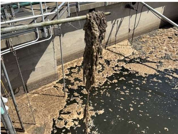
Rags on SBR level pressure transducer
