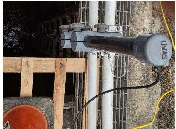
UVAS Probe in wet well
