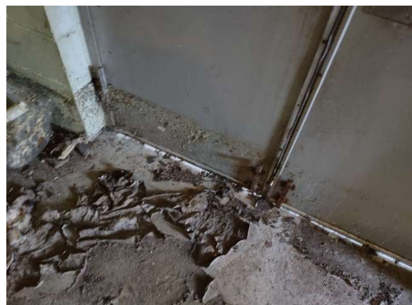
Flooding waterline in Hyco room
