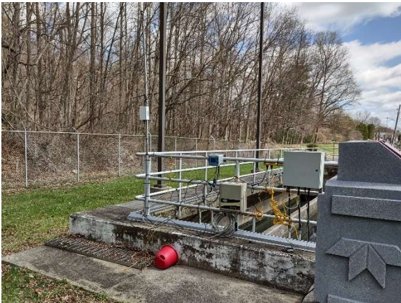
Effluent probe controller & telemetry
