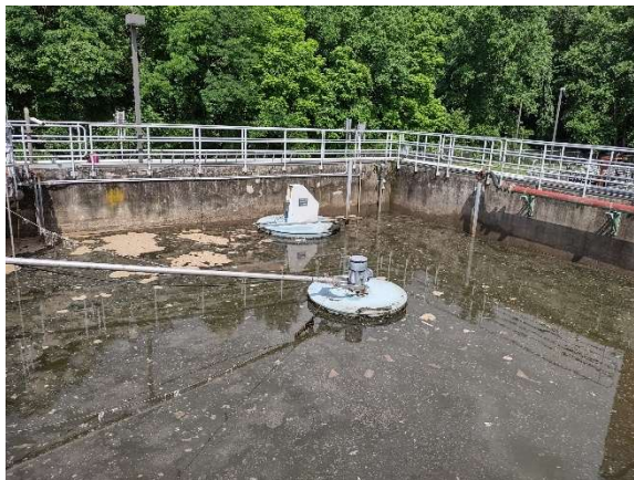
Photo 1: View of Lykens SBR at the start of decant phase.
