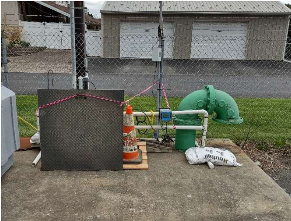
Influent Pump Station w/UVAS Probe
