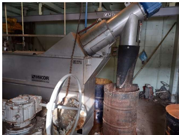
Photo 3: Hycor Preliminary Treatment Unit
