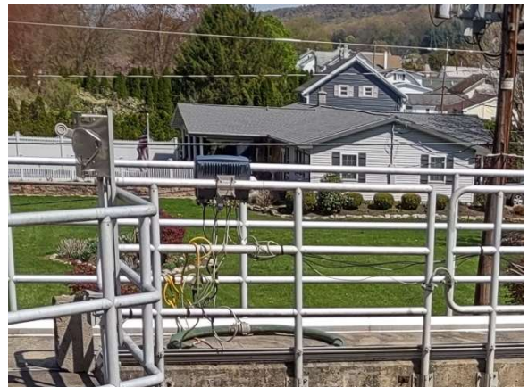
Upper probe controller for SBRs
