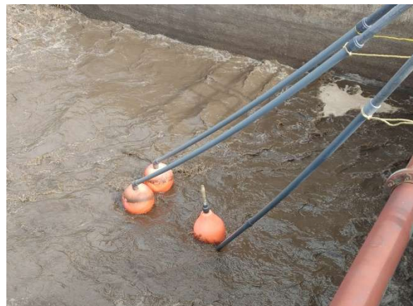
Broken probe mount due to turbulence.
