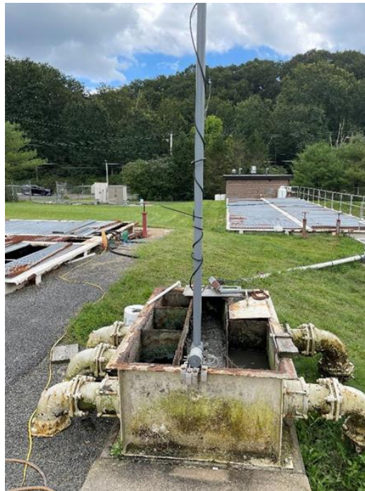
Figure 3: Photo of UVAS-2 continuous monitoring probe installation location at NESJMA WWTF flow splitter box from September 15 th through October 11 th , 2023 (end of study).
