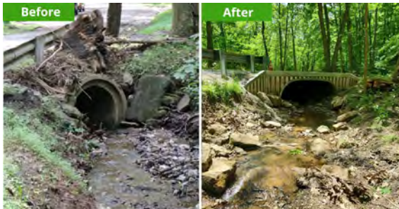
A culvert replacement in Sewickley Heights Borough allows for the passage of fish and reduces streambank erosion.
