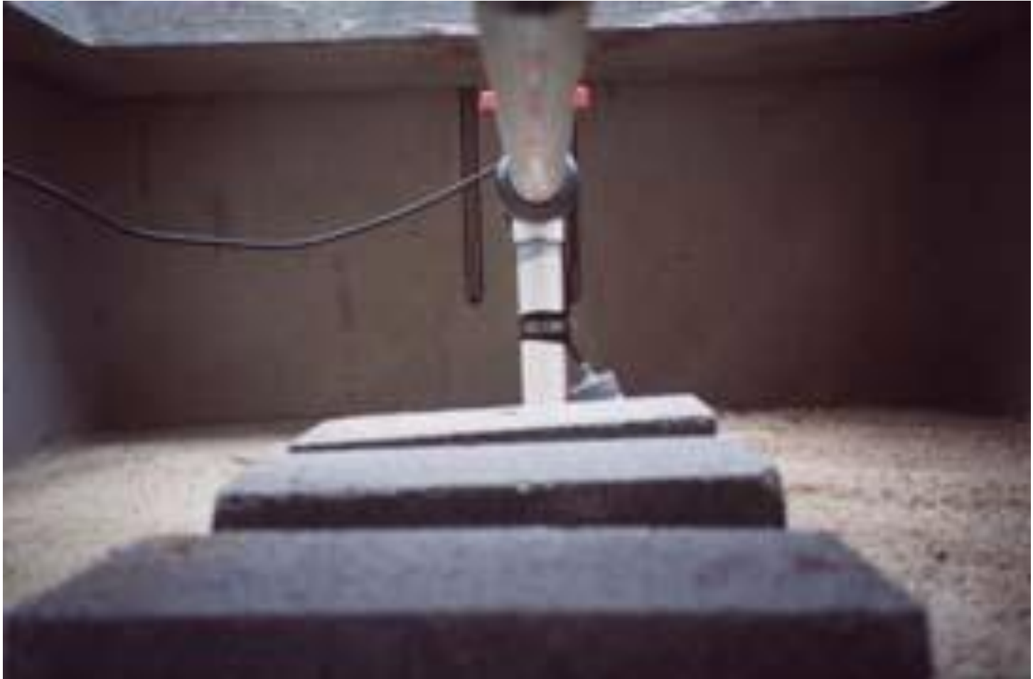
Interior view of sand filter.
