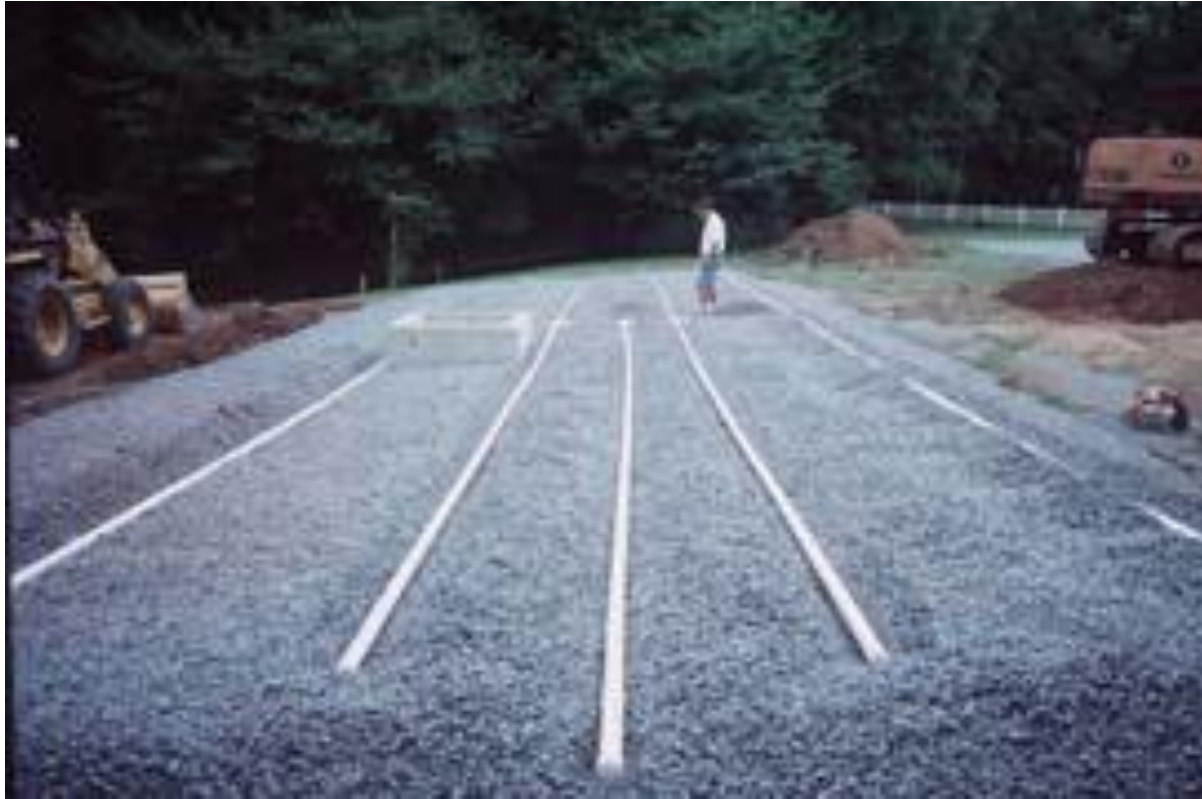
Pressure distribution pipe within bed area.
