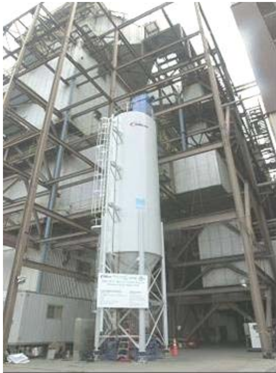
Activated carbon silo
